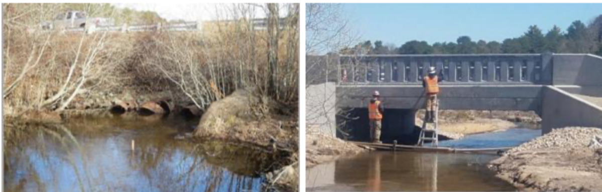
John Parker Road stream crossing before and after restoration activities, part of the Coonamessett River. (Photo from the Municipal Vulnerability Preparedness packet .)
