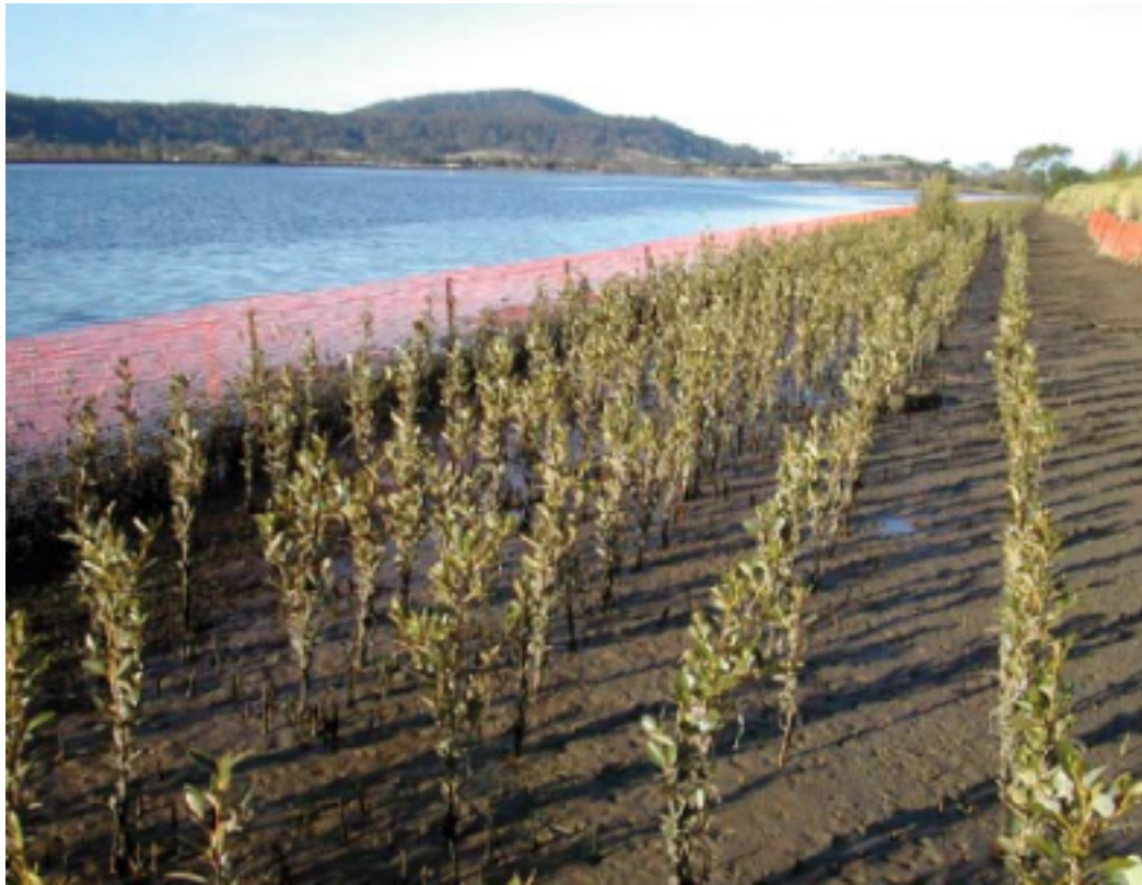
Fig. 1a. Typical mangrove rehabilitation works using Grey Mangrove seedlings on the Shoalhaven River, south coast of New South Wales. A similar method can be applied to the subject site at the Parramatta River.
