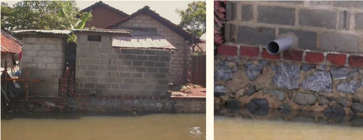
Figure 4. Pipes discharge faecal material directly into the estuary.
